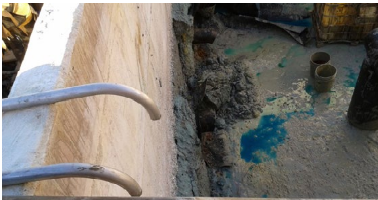
Dilapidated concrete acid tank (in disrepair due to many years of exposure)
